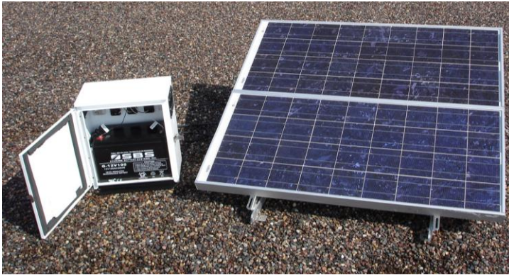
Figure 38: Solar Cell Power System
