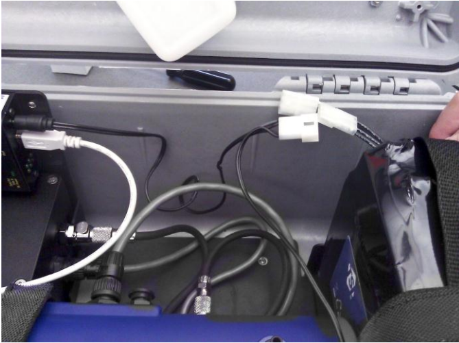
Figure 36: Internal DC Power Connections
