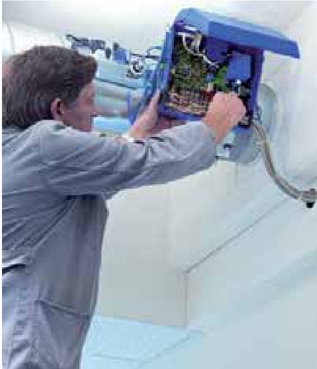
Commissioning of EASYLAB
